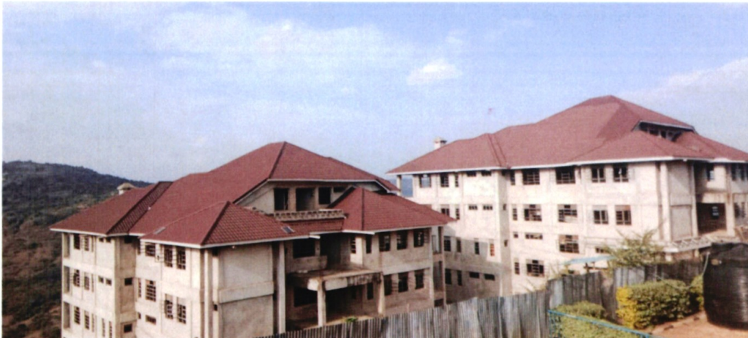
Photo 18: CWSK Murang'a: Aerial view of a section of Integrated child and family centre
