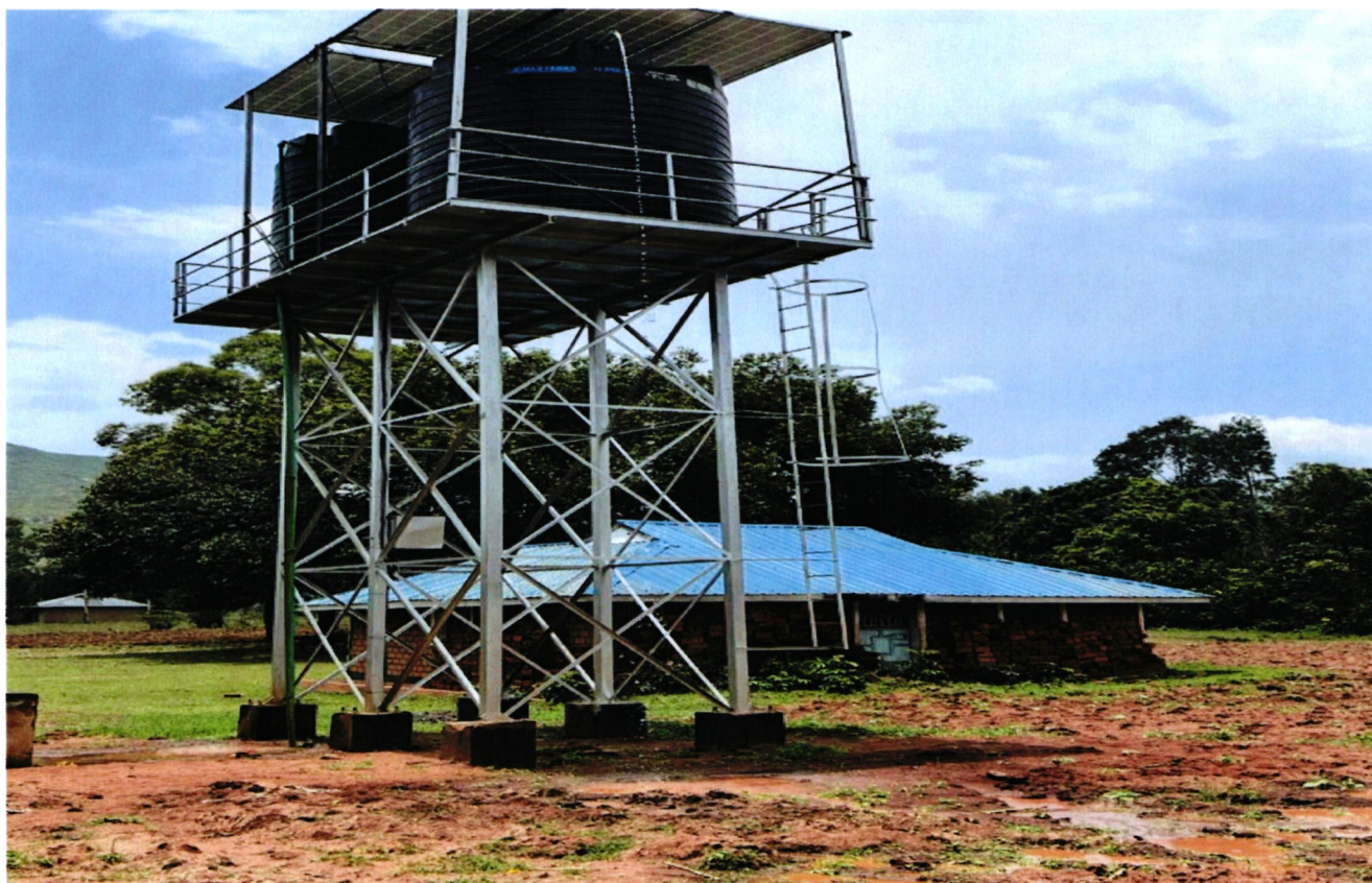
An installed water tank
