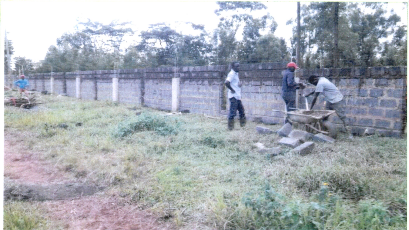
Figure 9: Construction of the College Perimeter wall to enhance security and safety of its property at Ksh 250M.
