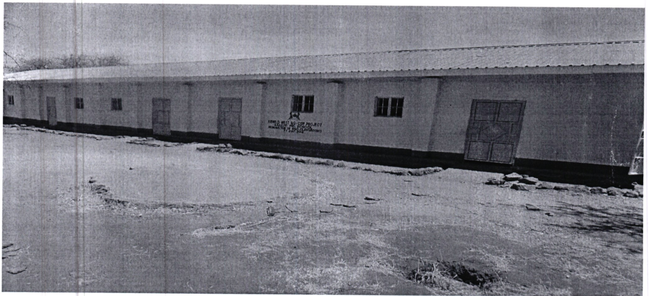
KAASUVI PRIMARY SCHOOL RENOVATION OF 6 CLASSROOMS (This involves putting new roof, doors, windows, flooring and painting at a cost of Kshs.1Million)
