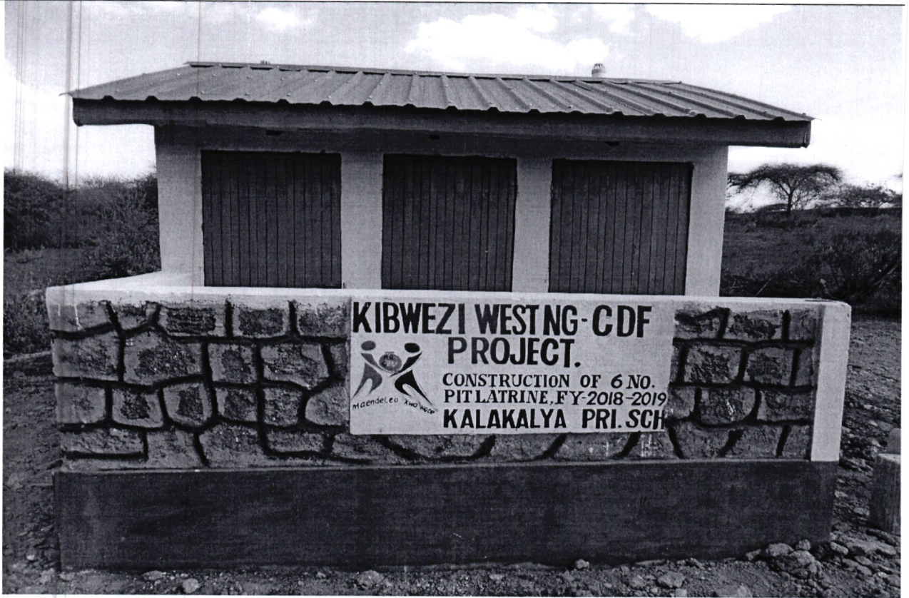
EMERGENCY TOILET AT KALAKALYA PRIMARY SCHOOL.
