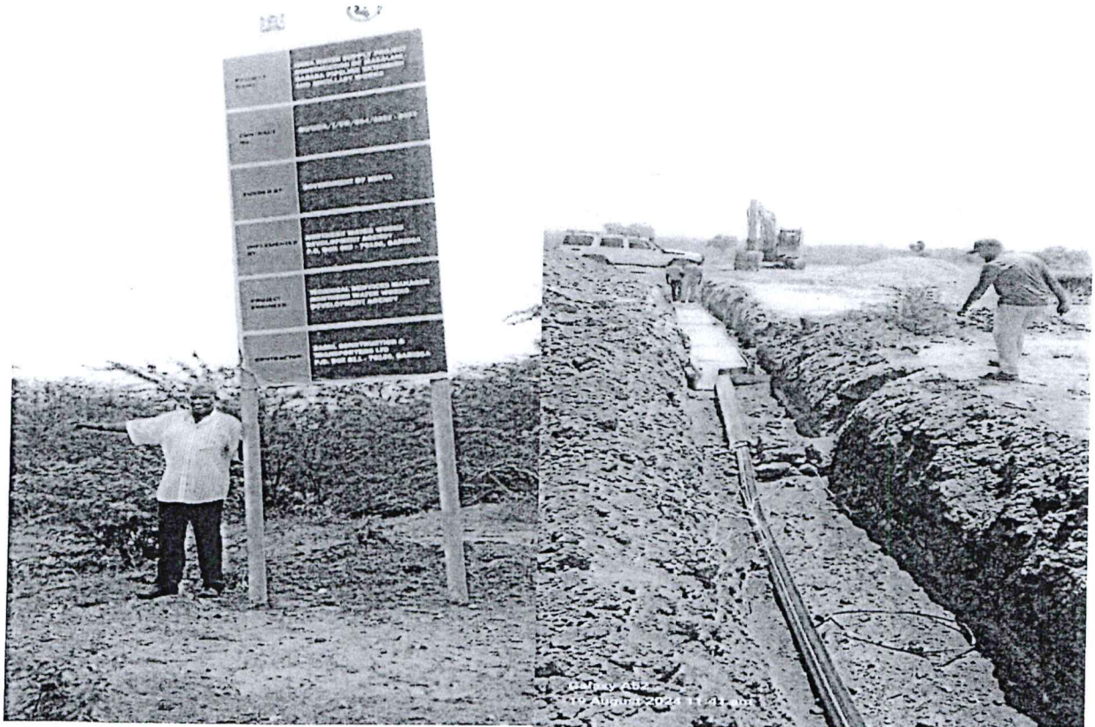
Figure 9: Masalani Gababa-Sign Board and Laying of the HDPE 110mm pipeline together with backfilling works.
