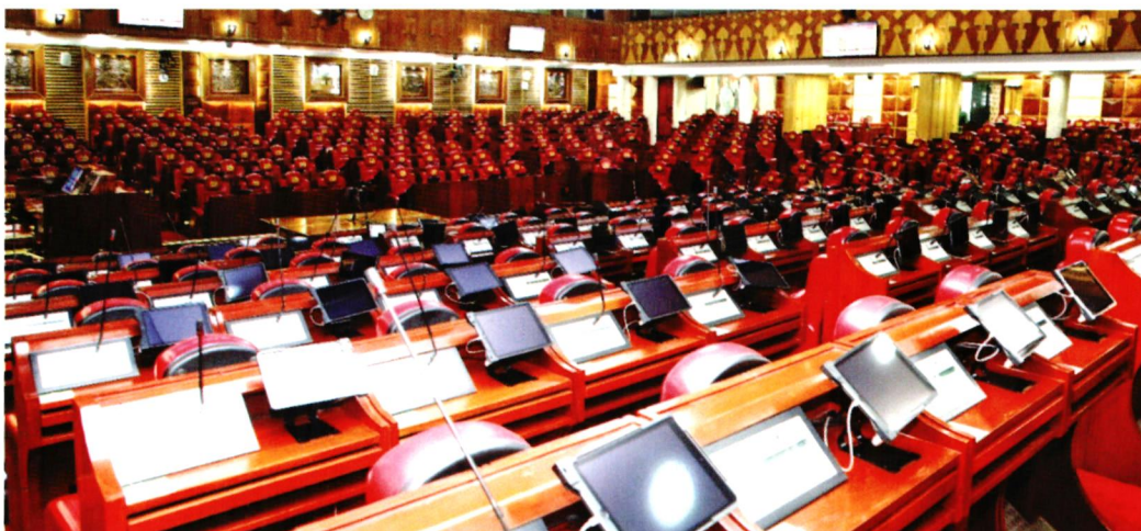
iPads installed in the National Assembly Chamber. The Order Papers, Committees Reports, and related documents are uploaded for ease of Members' reference
