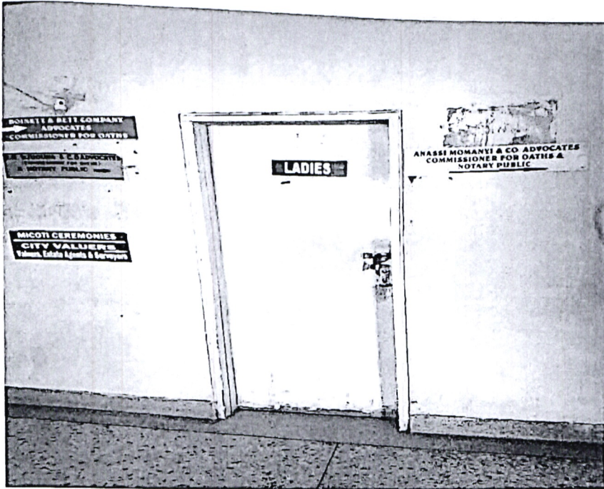
Photo showing state of the washroom doors.
