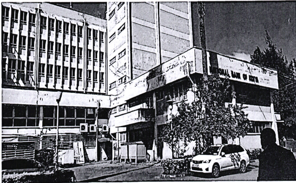
Photo showing view of the building from KVDA side and the state of external walls.
