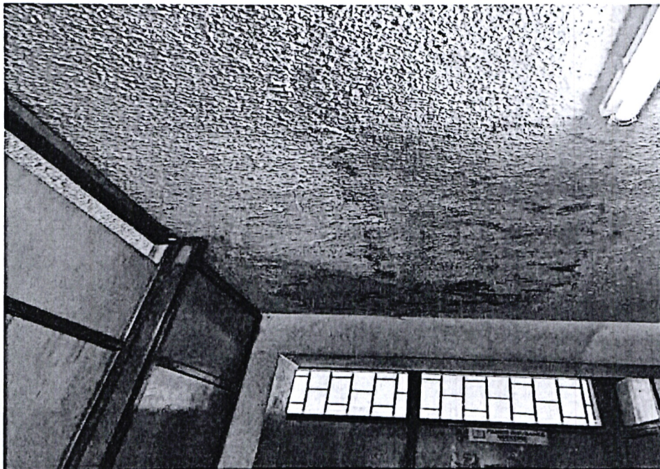
Photo showing water leakage from the concrete roof slab.
