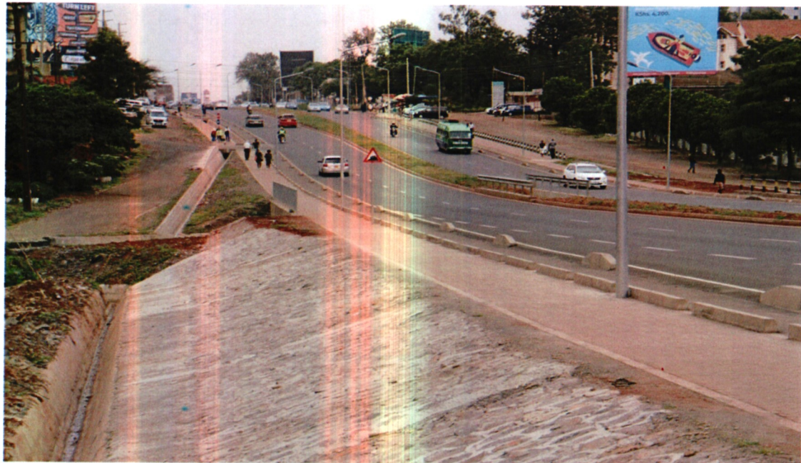
Figure 1: A completed section of Ngong Road Phase one in Nairobi county showing traffic separation
