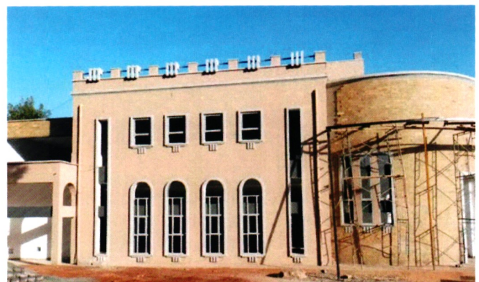
Construction progress of the Moot Court at the PTI, Loresho campus, Nairobi. Completion is set for Mid 2022.
