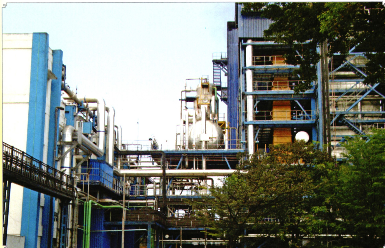
Cogeneration plant in Mumias Sugar Company
