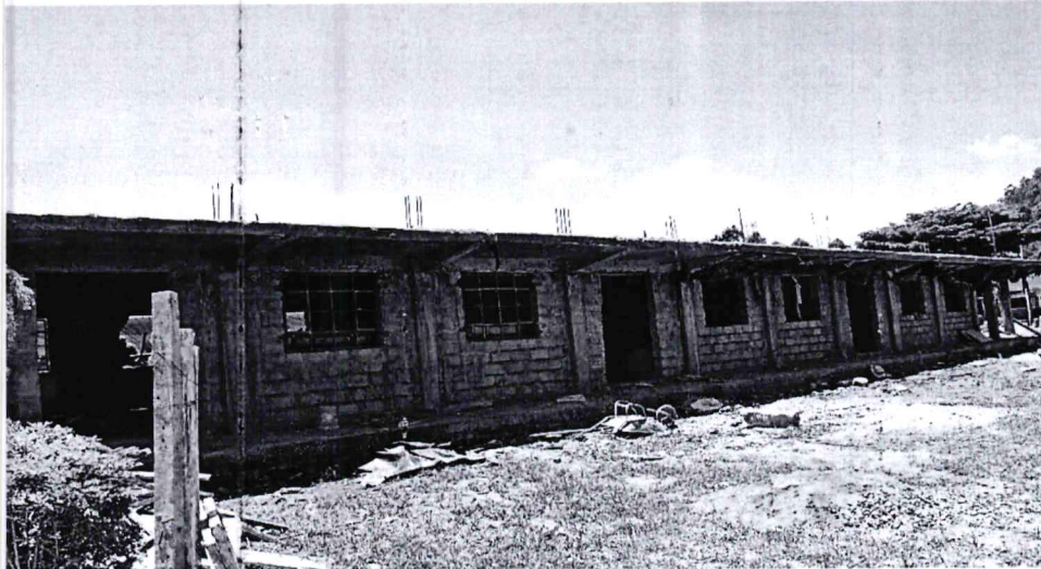
Construction of a storeyed 6 classrooms block at Maua Girls Secondary School (Phase I)
