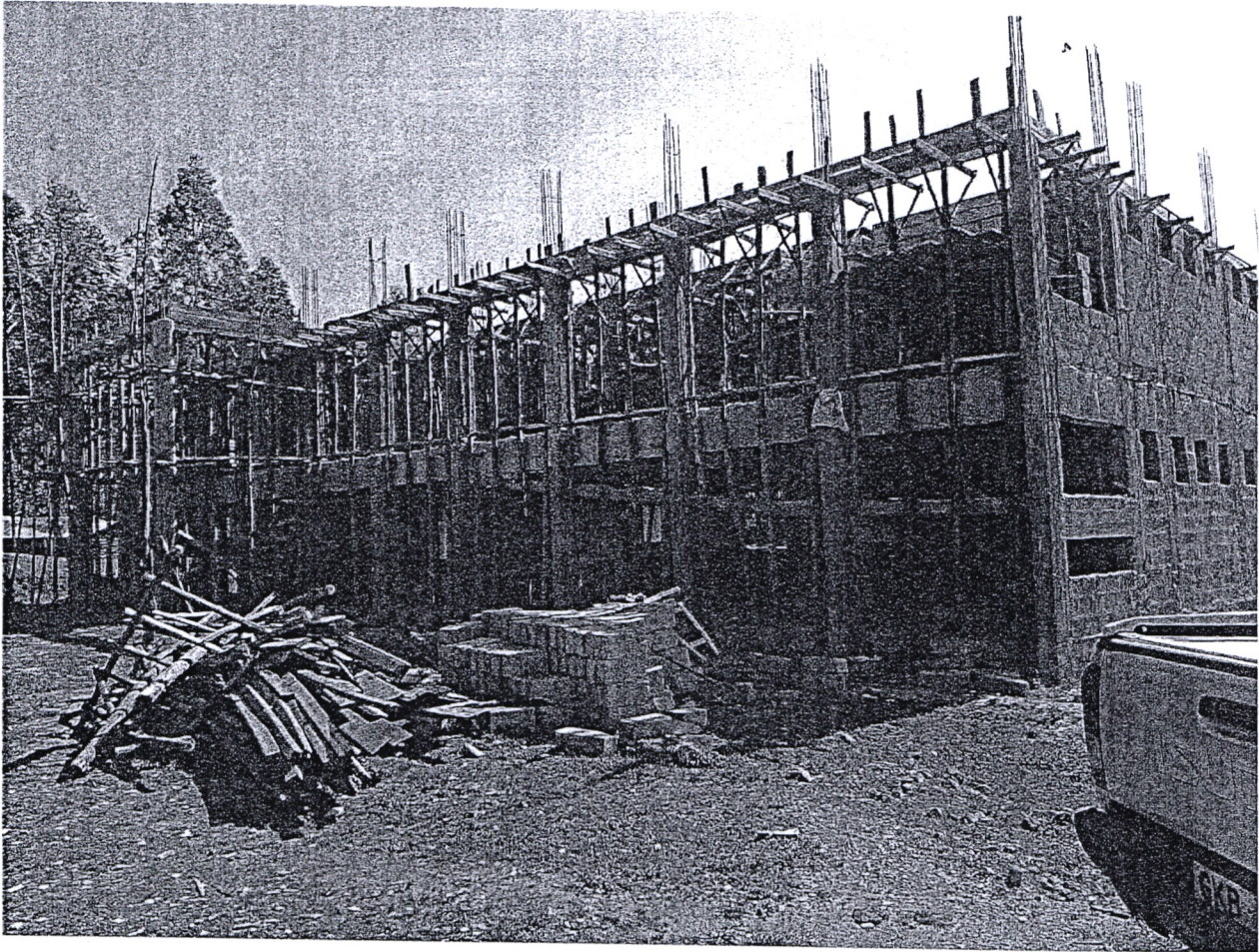
FIG. 02 ONGOING CONSTRUCTION OF MATUNGU KMTC ADMINISTRATION BLOCK & CLASSES Matungu KMTC project is the Constituency flagship project. So far ground floor is almost complete fitted with doors and window pens. Similarly ground floor has not been painted yet. 1 st floor has recently been casted with the upper slab and construction work is on-going. Recently NG-CDFB visited the project on normal audit evaluation and their recommendation was positive. After completion of the project FY 2022/2023 the project will have high economic impact within the Constituency.
