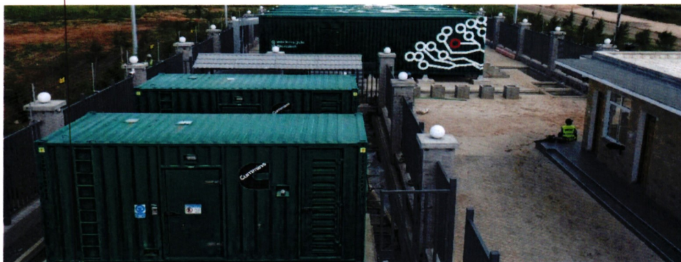
Phase 1 Data Centre
