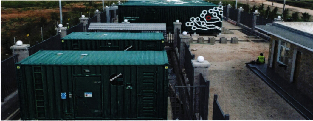
Phase 1 Data Centre
