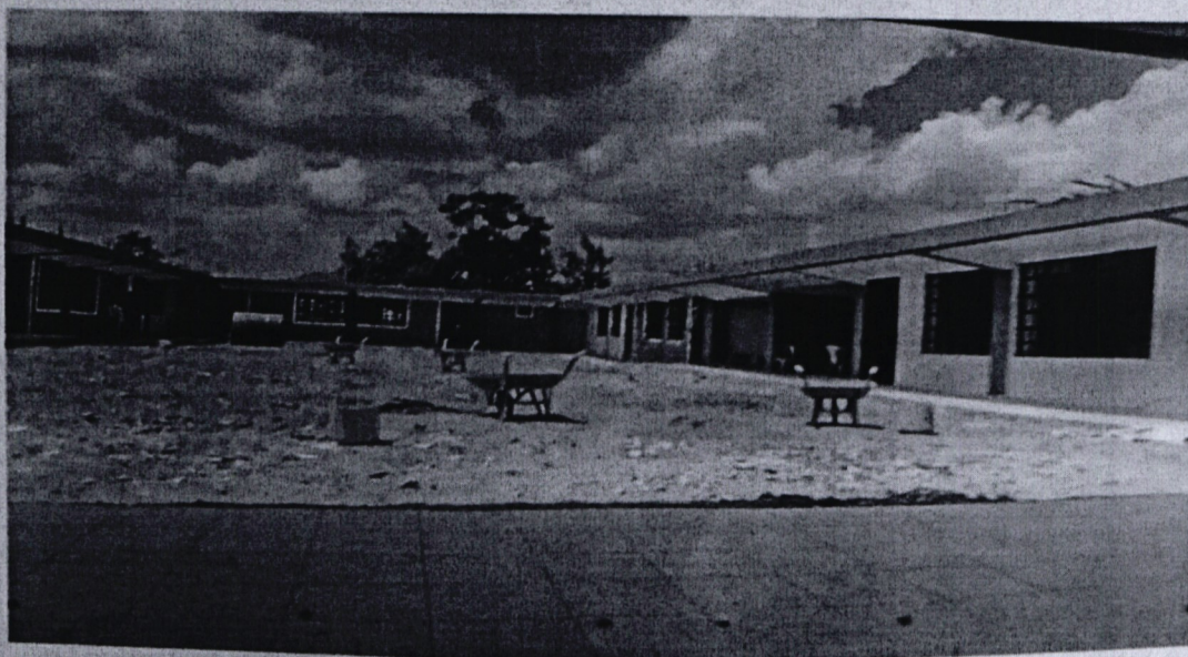
Project Name: Sisenye Mixed Secondary school Activity: Construction of a storey building( Phase 1: Construction of ground floor to completion)
