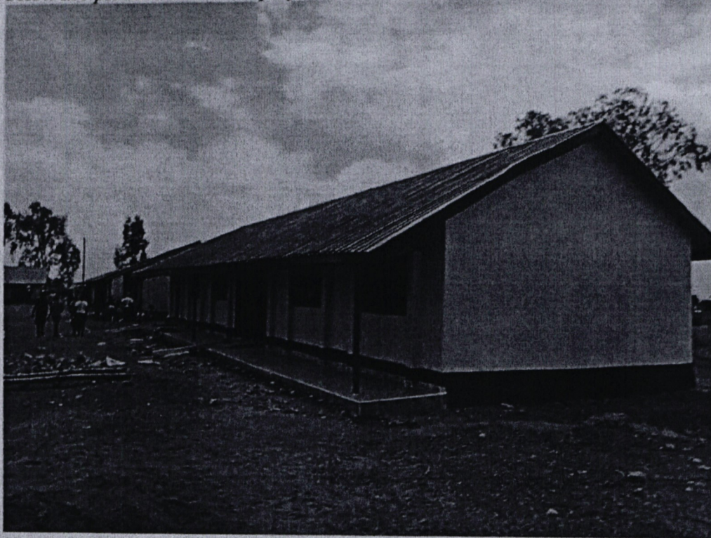
Project Name: Igigo Primary school Activity : Renovation of two classrooms to completion.
