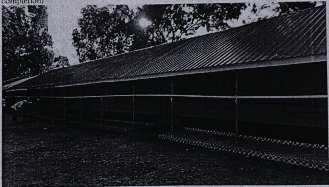
Project: Budubusi Primary school Activity: Renovation of four classrooms and office to completion
