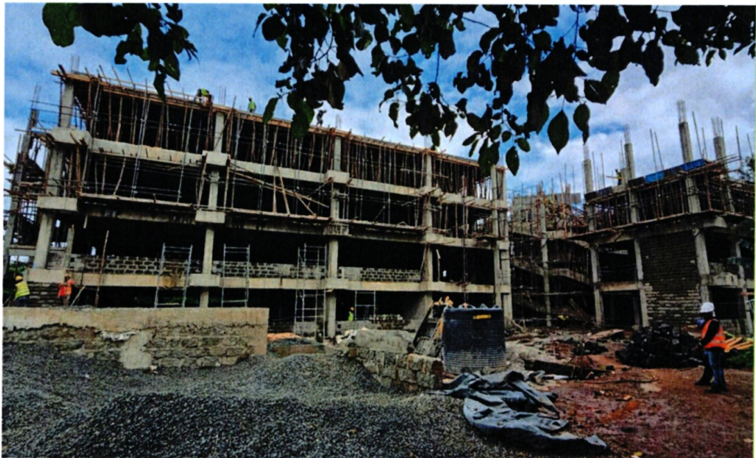
Site inspection of a building under construction in Kirinyaga County to ensure compliance with engineering standards
