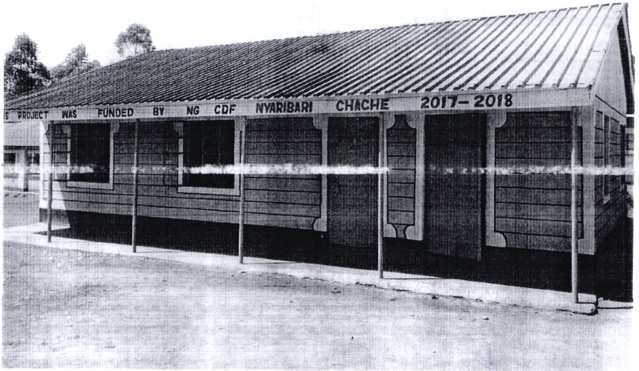
Fig 3: Construction of one classroom at Nyosia Primary School fully funded by Nyaribari Chache
