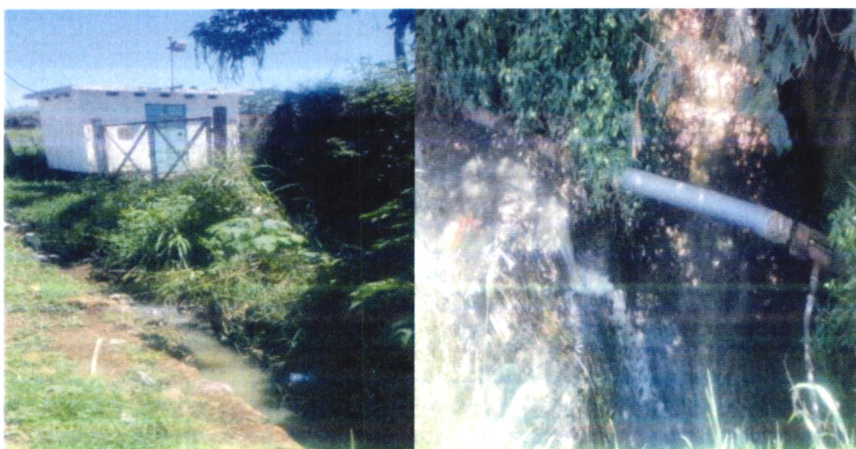
Plate 1: Waste water flowing into the environment from Kendu Lane pump Station
