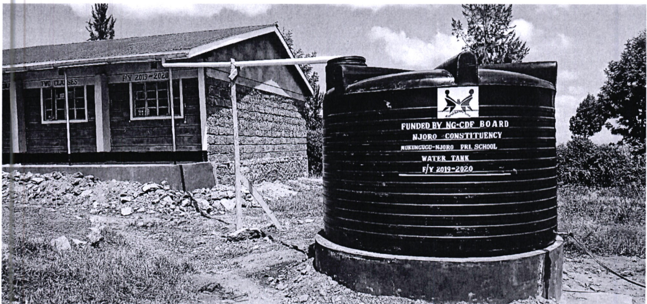
Mukungugu Primary School- Construction of 2 classrooms and Installation of a 10,000 ltr water tank
