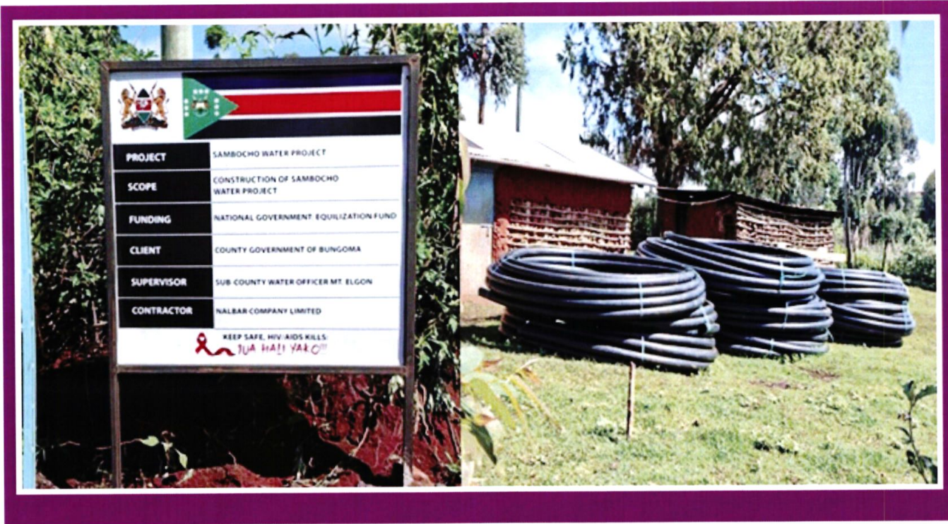
Picture 9 : Publicity Signboard and water pipes for the Sambocho water project
