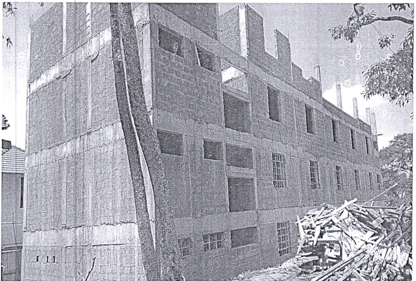
Figure 3: Ongoing Construction of 3 Floors (400 student's capacity) Modern Dormitory Block at Nairobi Milimani Secondary School.
