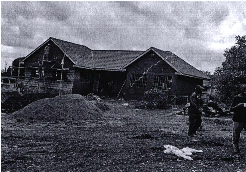
KENYENYA ACC'S OFFICE AND SMALL CLAIMS COURT. -Ongoing construction of Kenya ACC office and Assistant chief's office
