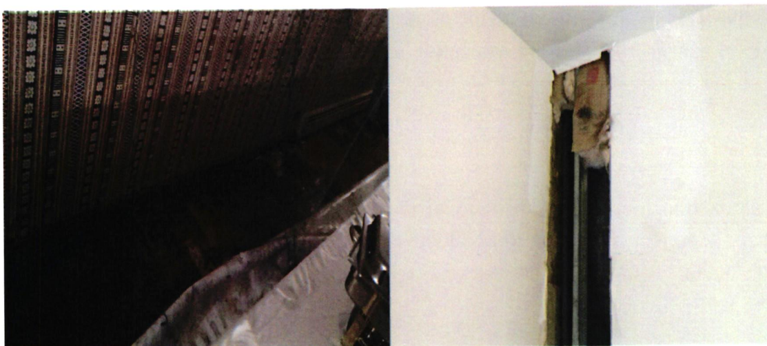
Sections of the dilapidated Kenya House in New York
