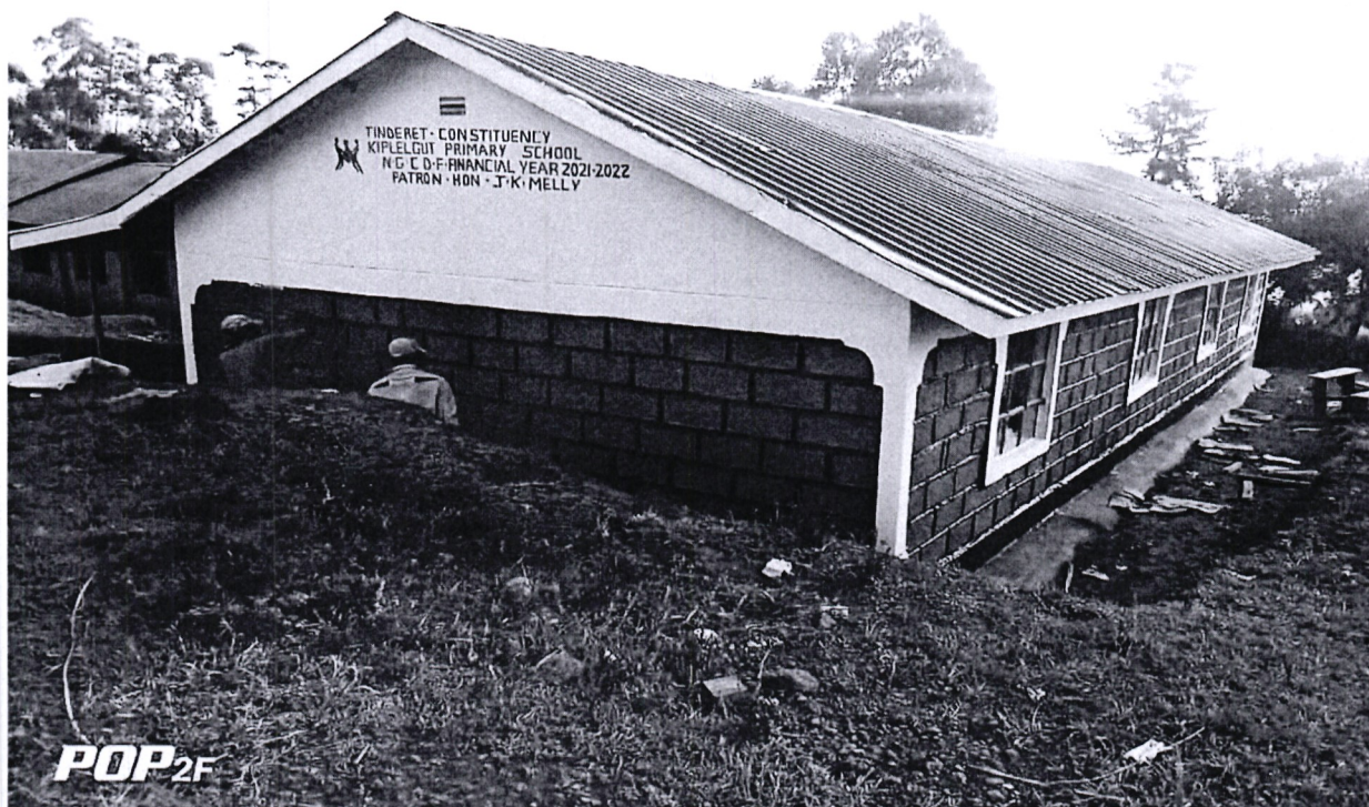
Kiplegut Primary School: Renovation of 2 classrooms (flooring, painting and fascia board) to completion.
