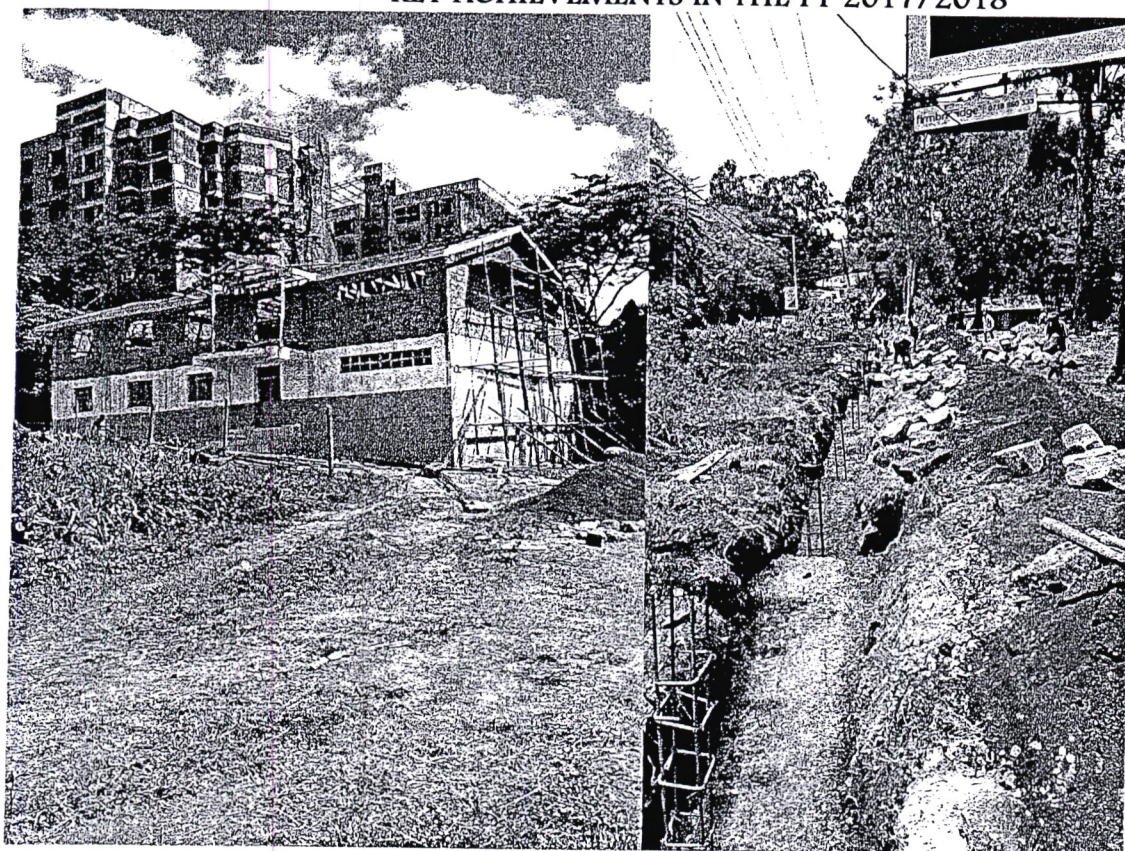
Fig 1: Construction of Dormitory on first floor at St. Georges Primary School and construction of PERIMETER wall at Nairobi Primary School respectively.
