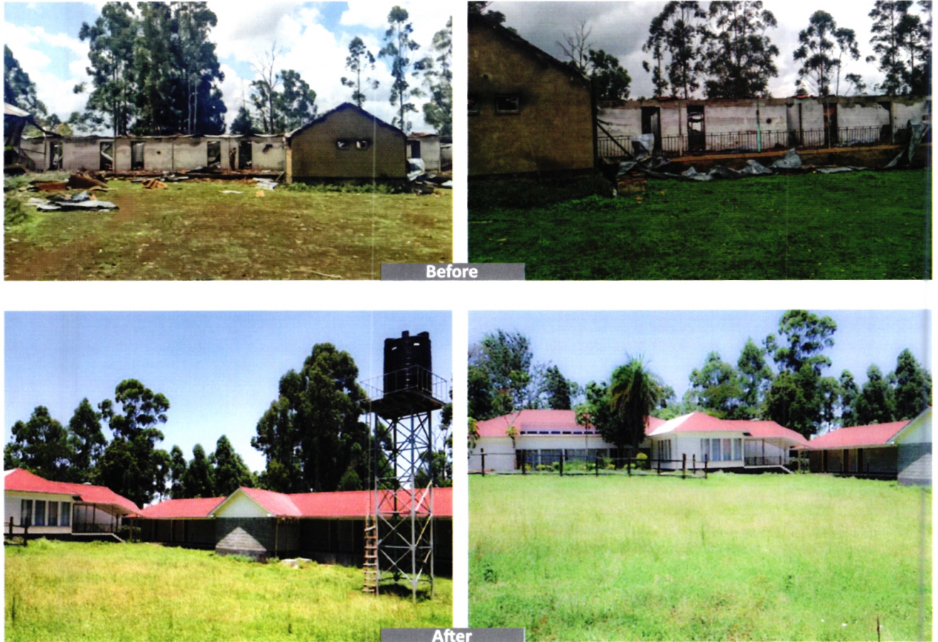
State of WOs & Sgts Accommodation before and after Completion of Renovation on 08 Oct 2019.
