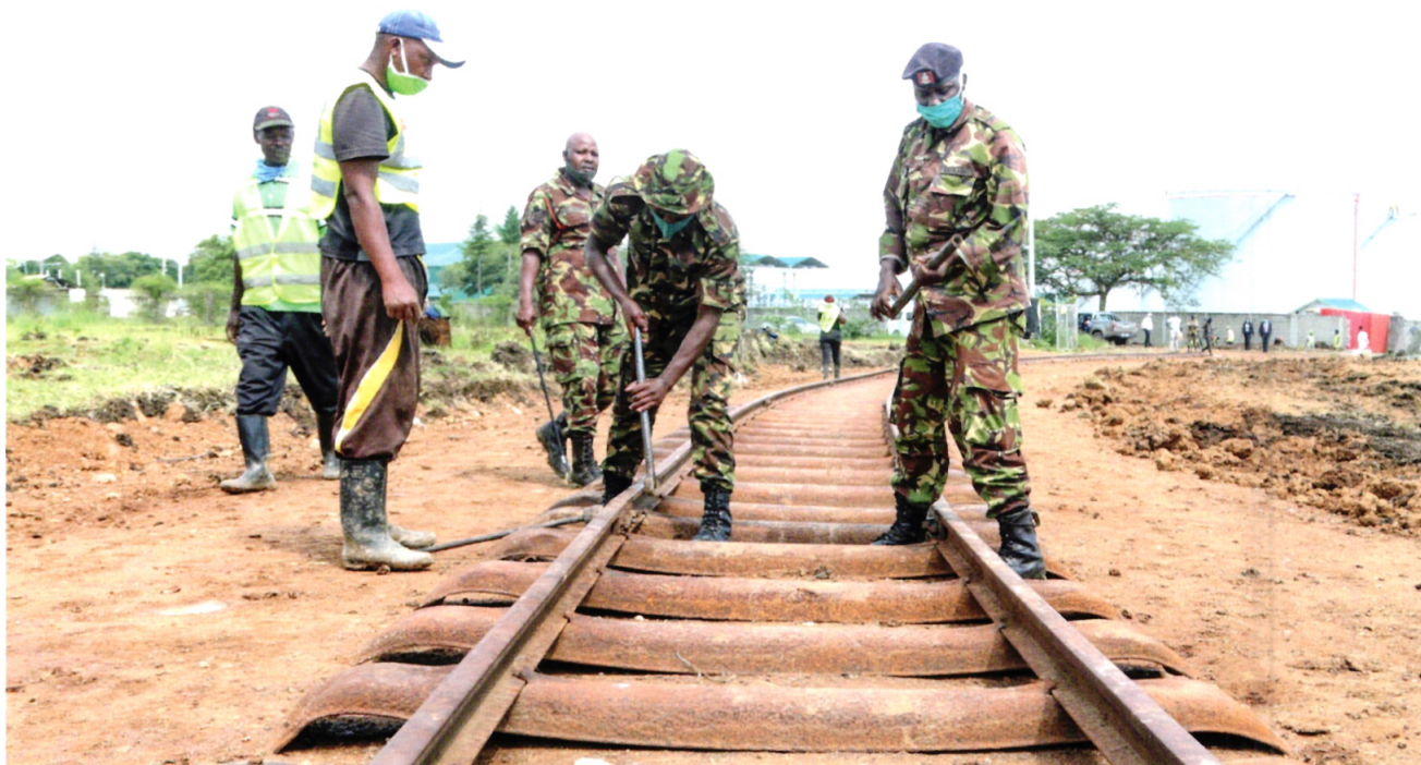
Kenya Army Corps of Engineers (KACE) soldiers rehabilitates the Thika-Nyanyuki Railway line.
