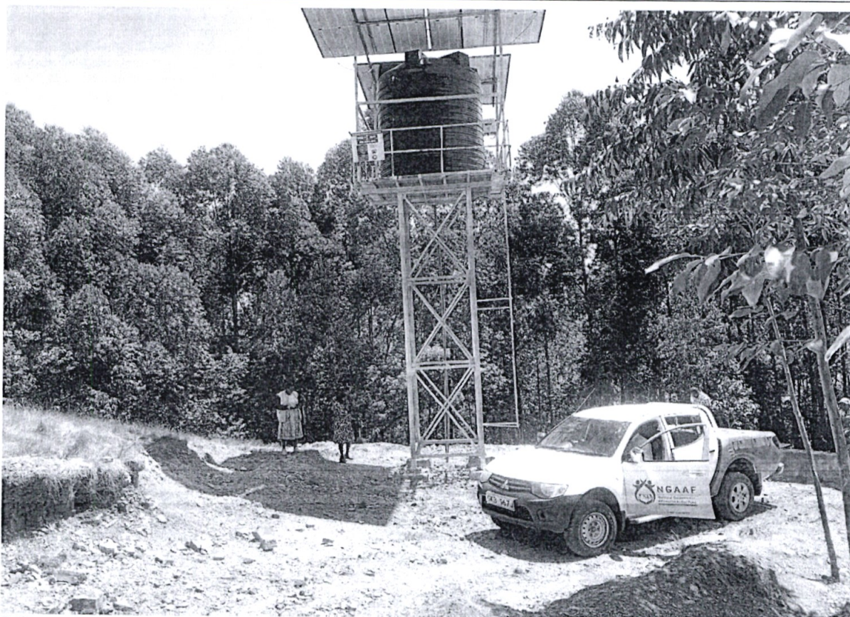
Drilling and equipping of borehole at Nyamage School, Bobaracho in Kisii County. The borehole will serve the school and neighbouring community members to access water
