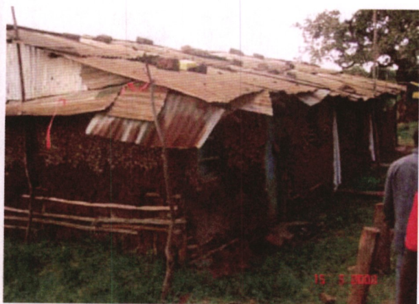
Dilapidated quarters for warders - Kisii Prison
