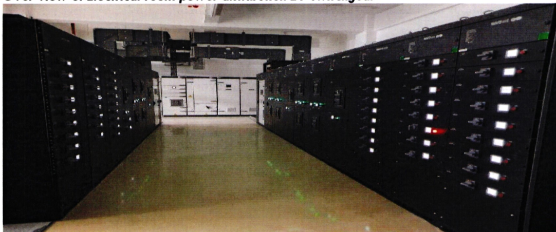
Over view of Electrical room power distribution LV switchgear
