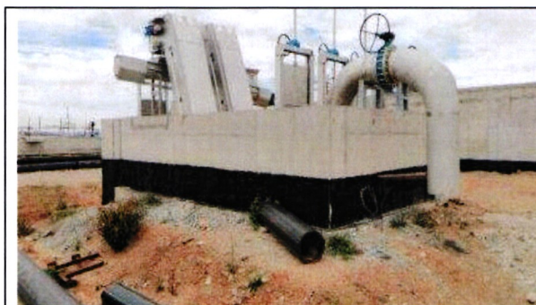
Preliminary Treatment - Mechanical installation
