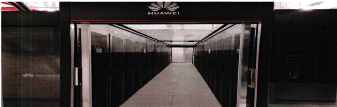
Data centre module 2000 installed
