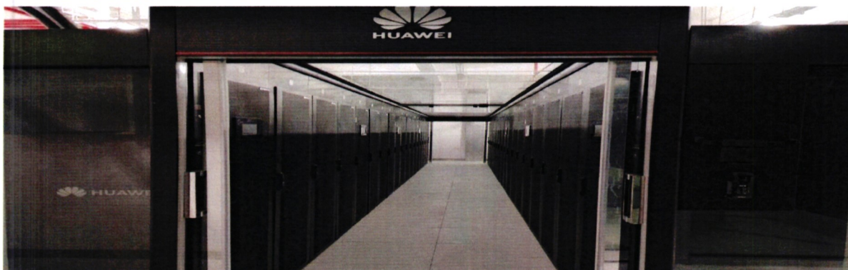
Data centre module 2000 installed
