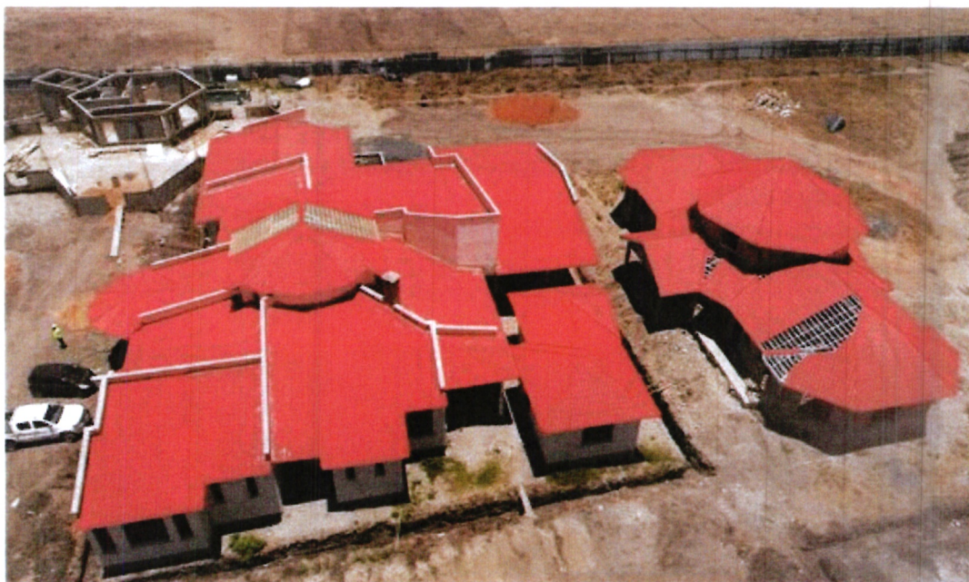
Ongoing construction of a bungalow, administration unit and kitchen/dining units at CWSK Joska Integrated Child & Family Centre
