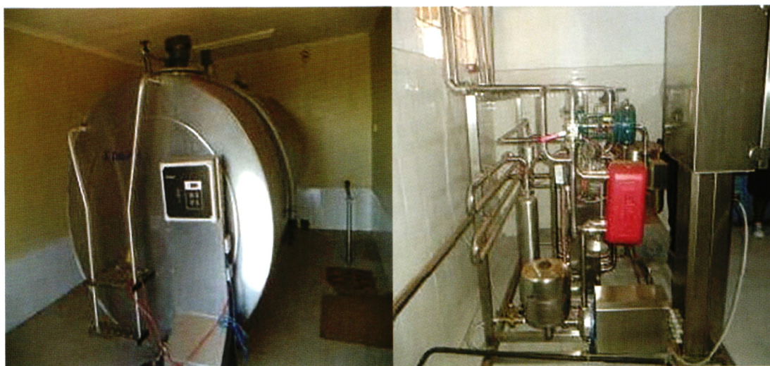
Newly installed 5000 litres milk cooling tank and pasteurization unit at Muguga Farmers' cooperative society, Kiambu County.
