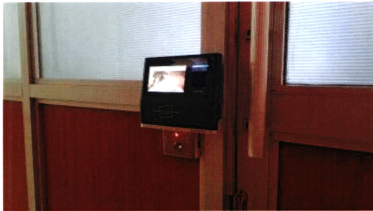
Biometric systems have been installed on all floors including the server room
