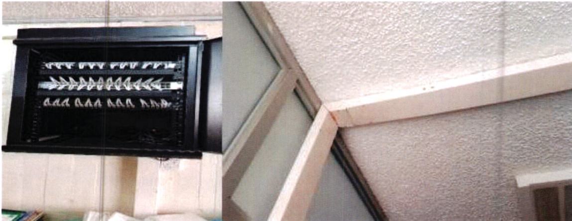
Structured cabling and trunking
