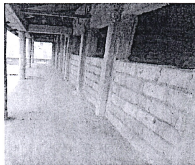
Figure 004: First floor corridor showing the Missing rails.
