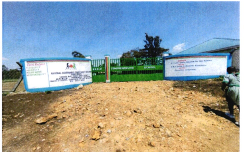
Akele Primary School - Fencing of School Compound and Installation of main Gate
