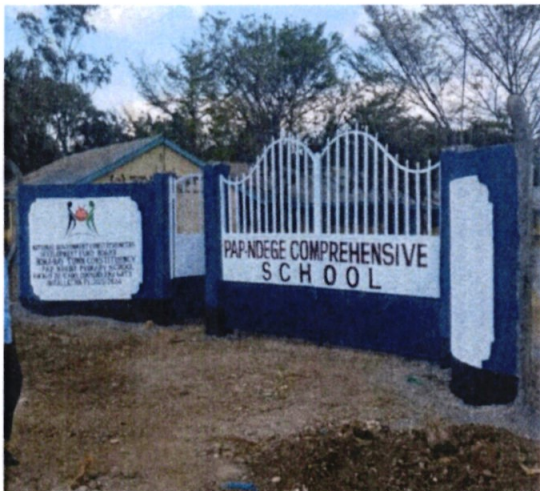
Pap Ndege Primary School -Fencing of School Compound and Installation of main Gate
