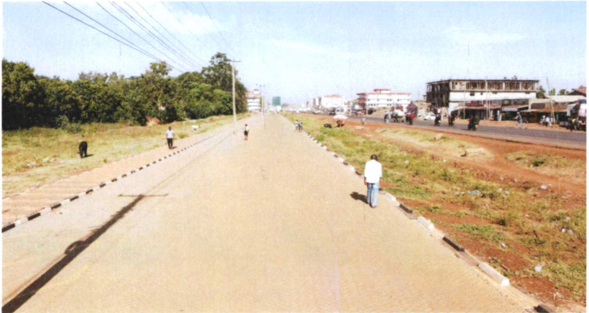
Newly laid cabro parking at the ATC (Agricultural Training Centre) in Busia
