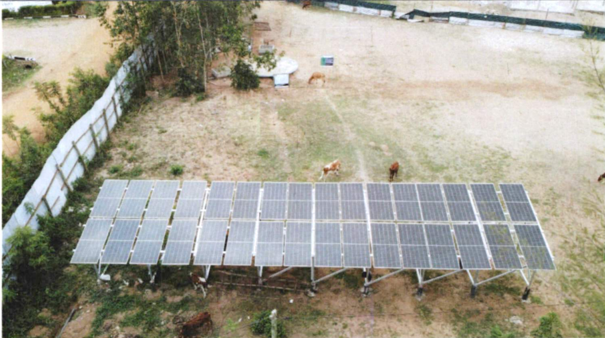
Newly installed solar panels at Kolanya Girls High School
