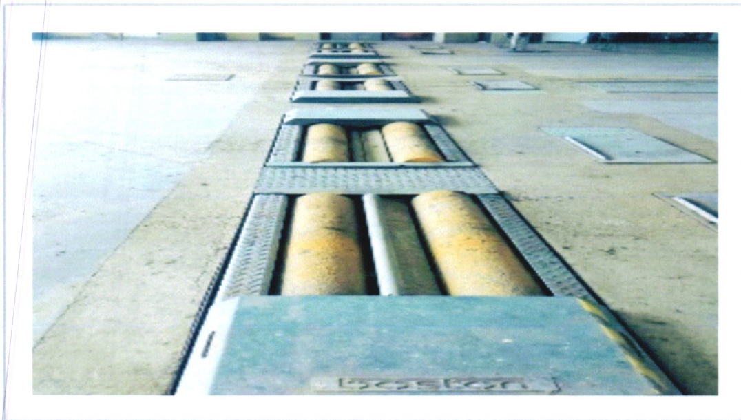
Motor vehicle test lanes installed in Motor Vehicle Inspection Centre Likoni Rd, Nairobi
