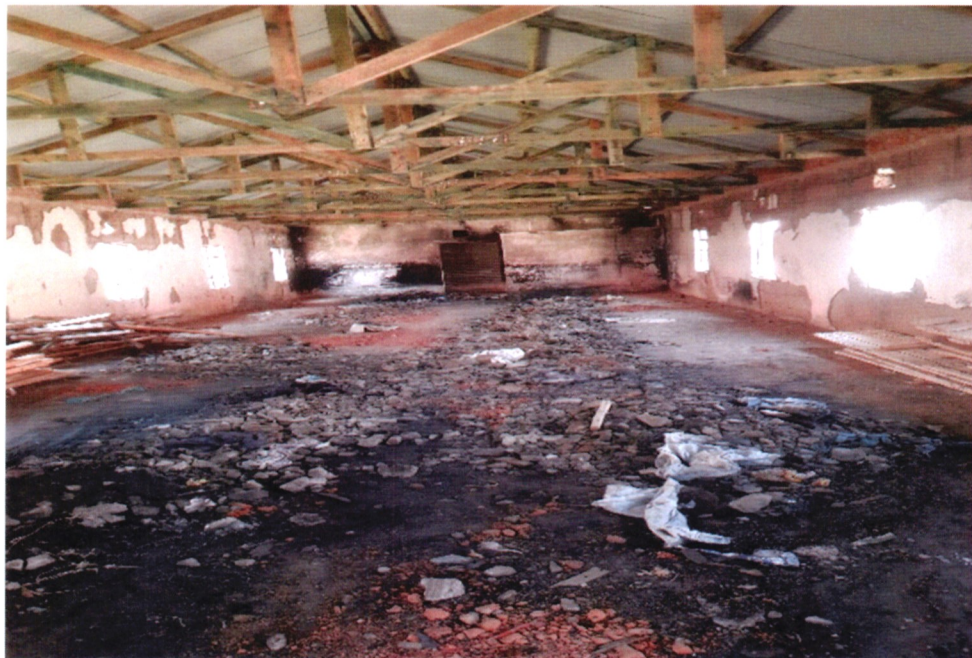
Source: OAG Staff physical verification of school buildings destroyed by fire
