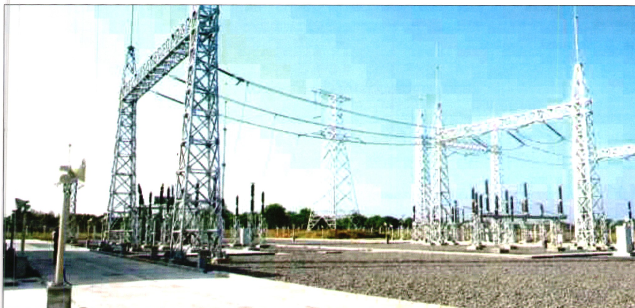
Lamu Power project
