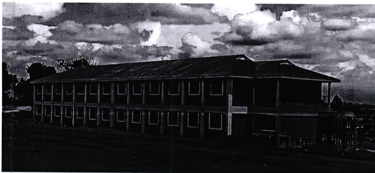
Caleb Amisi centre of excellence construction of 8 classrooms block, F/Y 2020-2021 Impact: to enhance transition from primary to secondary school.
