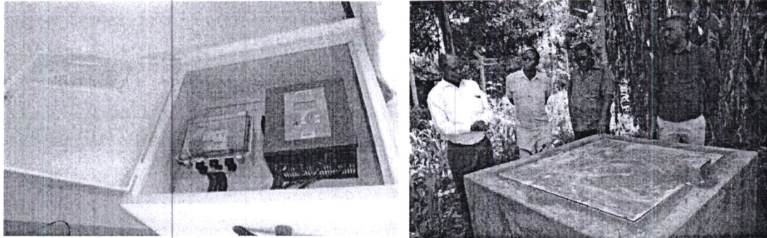
Picture 7: The Ipali Water tank in West Bunyore ward water tank
