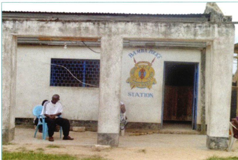
Bamba Police Station lacking a roof
