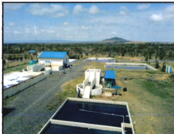
Effluent Treatment Plant aerial View
