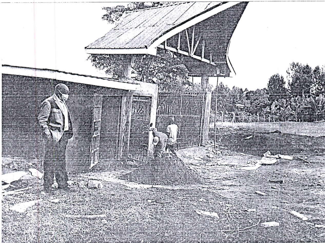
Fig 1.6 - Handege Primary School - Construction of gate with watchman cubicle and chain-link fence FY 2020-2021
