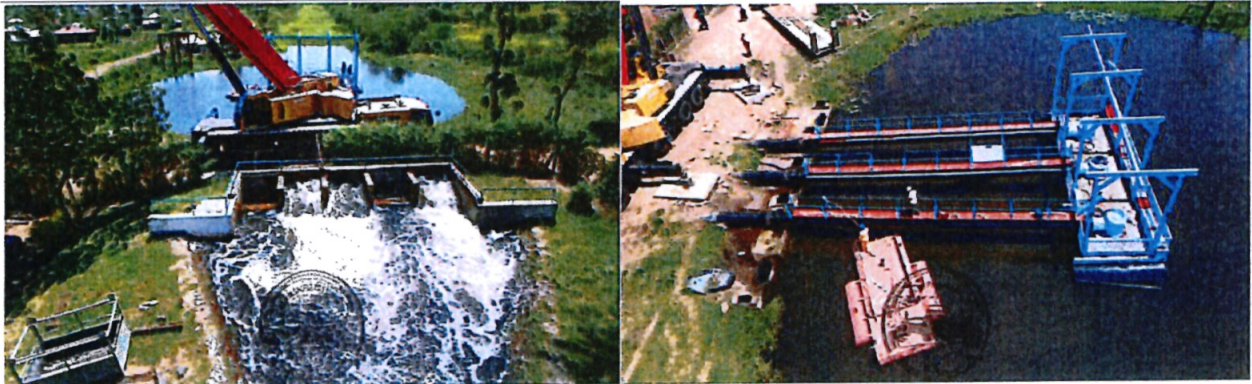
National Irrigation Authority: Kano Irrigation Pumps
