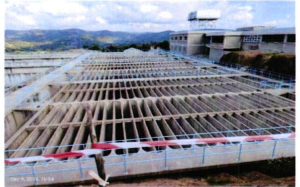
Flocculation Basin in Water treatment in Maruny (siyoi) Dam, Kapenguria water project
