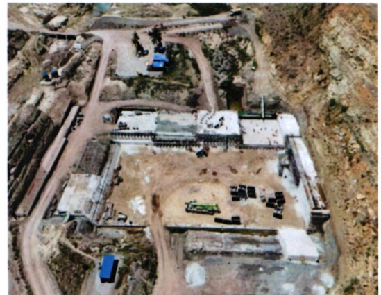
32m high Intake Tower and Diversion Channel in Muruny (siyoi) Dam, Kapenguria water project
