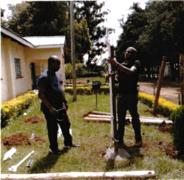
Installation of Automatic Weather Station in Teremi High School
