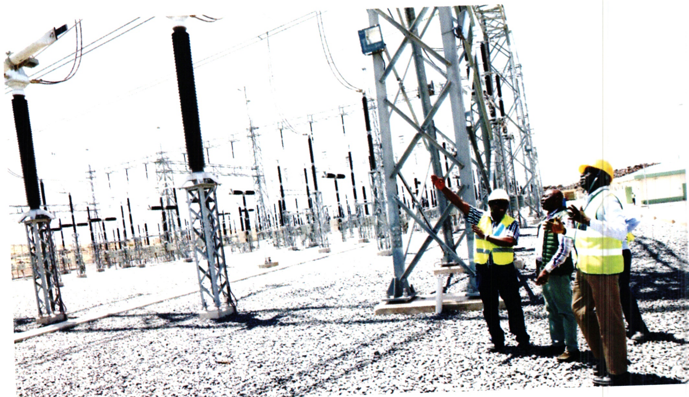
Loyangalani Transmission Line
