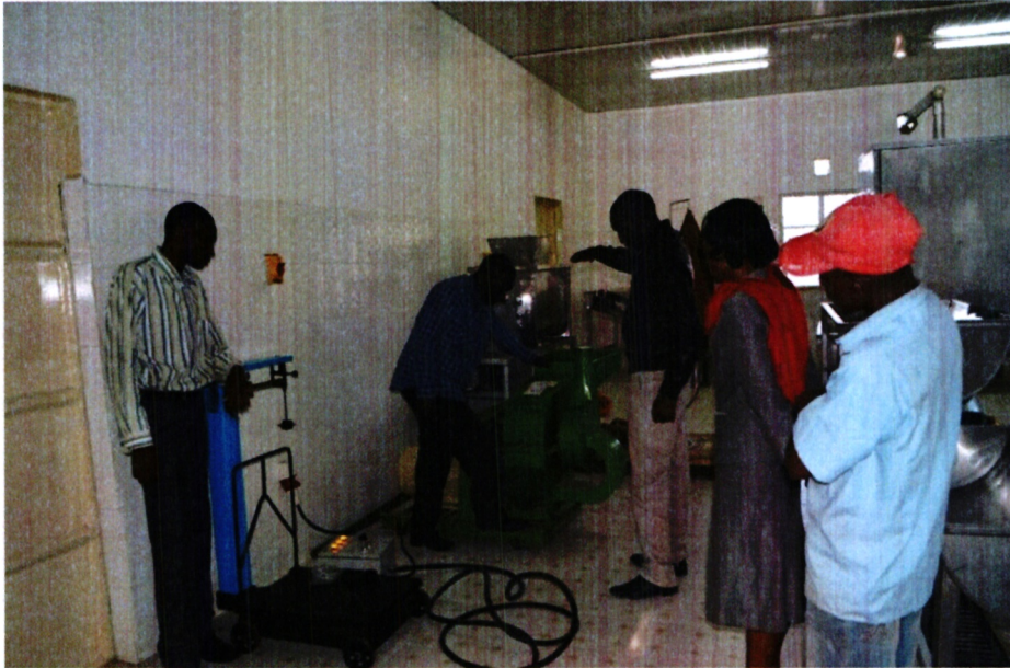
Photo 1: Installation of new machinery in one of the NETFUND supported Incubation businesses
