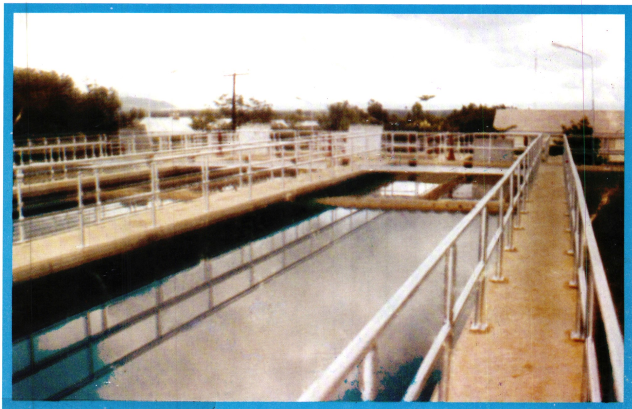
MASINGA WATER SUPPLY TREATMENT WORKS
