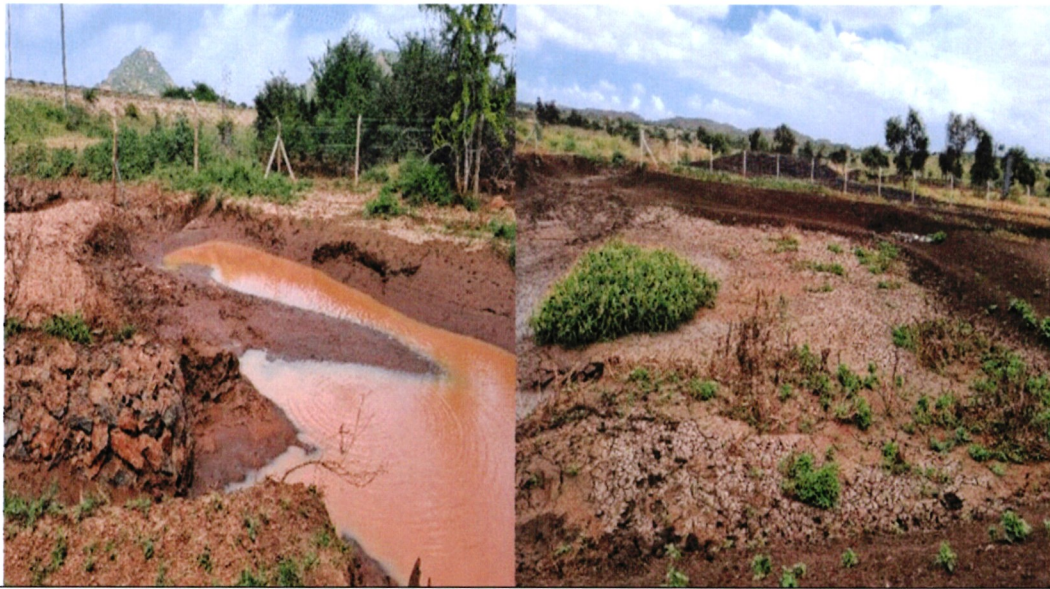
Left to right; Syomithumo and Nkoroshon water pans showing silted silt traps respectively. Source: Photos taken by auditors on 25 January, 2022 and 31 January, 2022 respectively.
