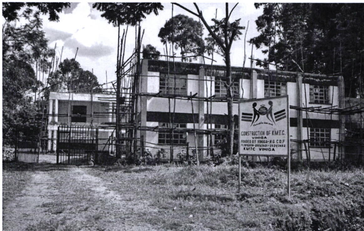
Figure 1: KMTC Vihiga - Ongoing Construction of Administration Block Phase II Statutory Compliance and Financial Obligations
